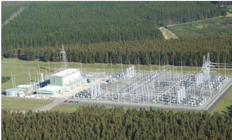
Basslink single circuit converter station and switchyard
