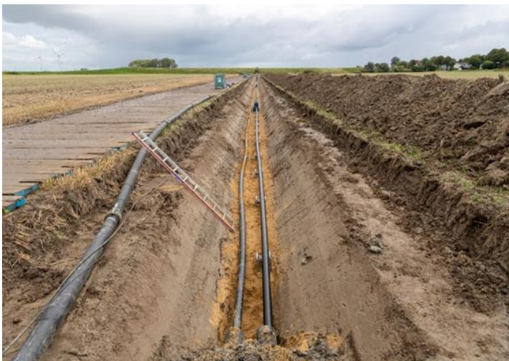
HVDC cable trench
