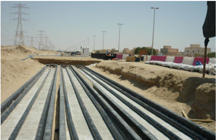
High-capacity single circuit cable trench
