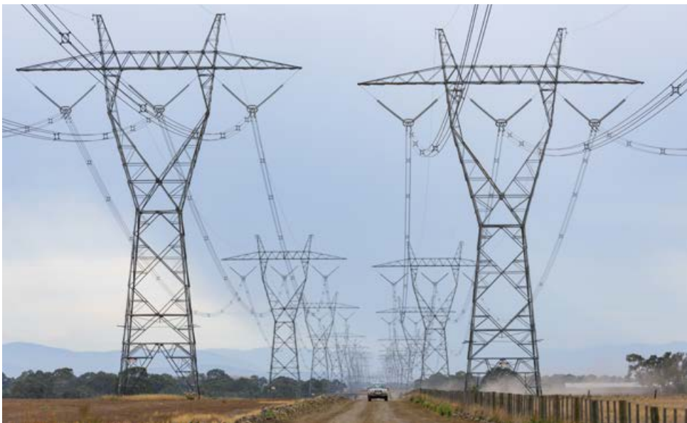
Single circuit transmission towers
